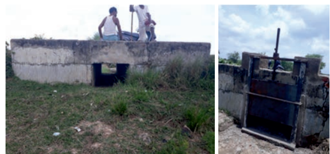
Views of a pond inlet before and after installation of a sluice gate to prevent backflow.
